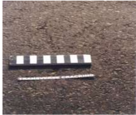
CRACKED ROAD (UNMODIFIED)
